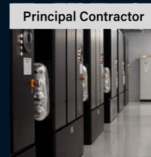
Data Centre, London
